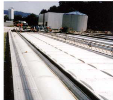
Abdeckung eines Sandfanges Covering of a sandpit
